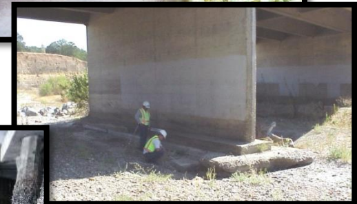
Degradation (below ground/water)
